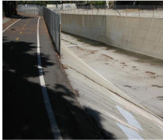
(b) Looking upstream away from confluence – transition to vertical walls and fencing
